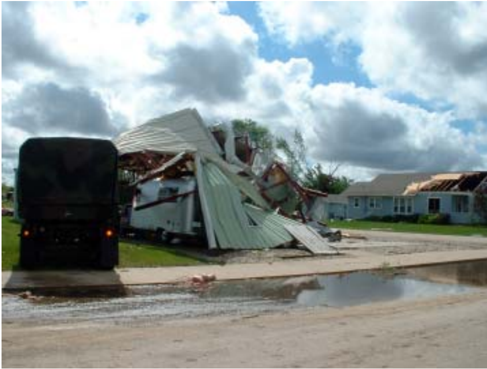
Looking southeast from the center of town. A garage destroyed in foreground and roof damage in the background. (F1).
